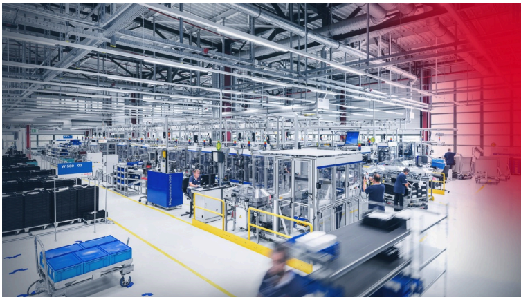
Bosch relies on the control system ctrlX CORE at its Blaichach plant. (Image source: Bosch Rexroth AG)
