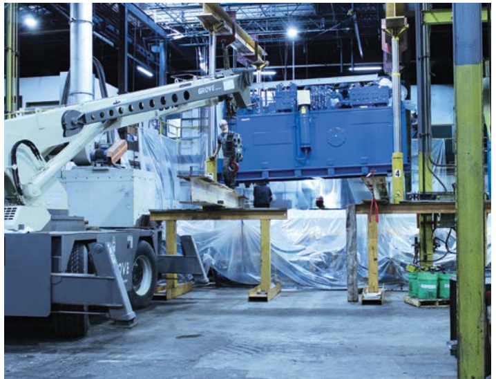
The power unit had to be carefully rigged into position above existing equipment.
