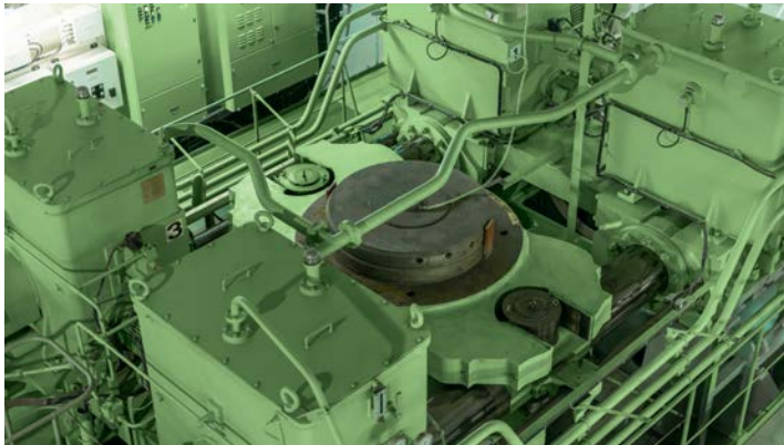
▲ Hydraulic rudder system on a container ship
