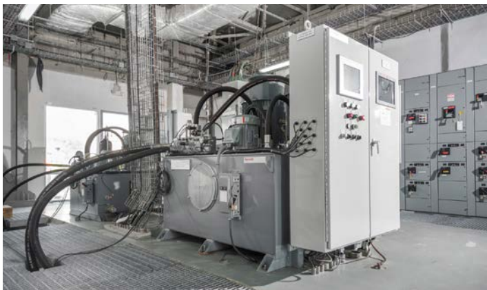
Hydraulic power units with stainless steel and flexible lines
