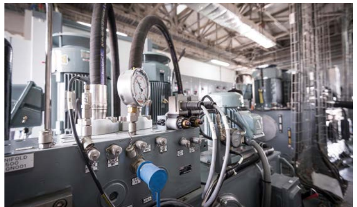
Control block of a hydraulic power unit with pressure gauge
