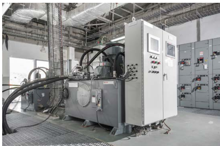
Complexity in applications or specification may require complex control packages nearly the same size as the hydraulic power unit. A well designed and built power unit not only achieves functional criteria but can also be an attractive addition to the production floor..
